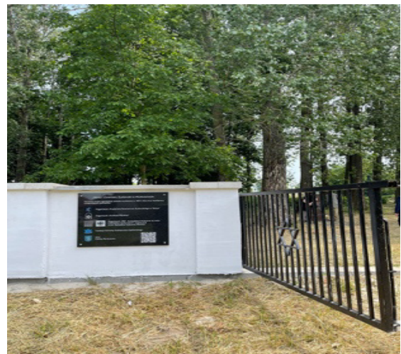
Figure 29. Markuszów Jewish Cemetery - new fence and wall around part of the cemetery; the remainder will be delimited with a plant hedge.
