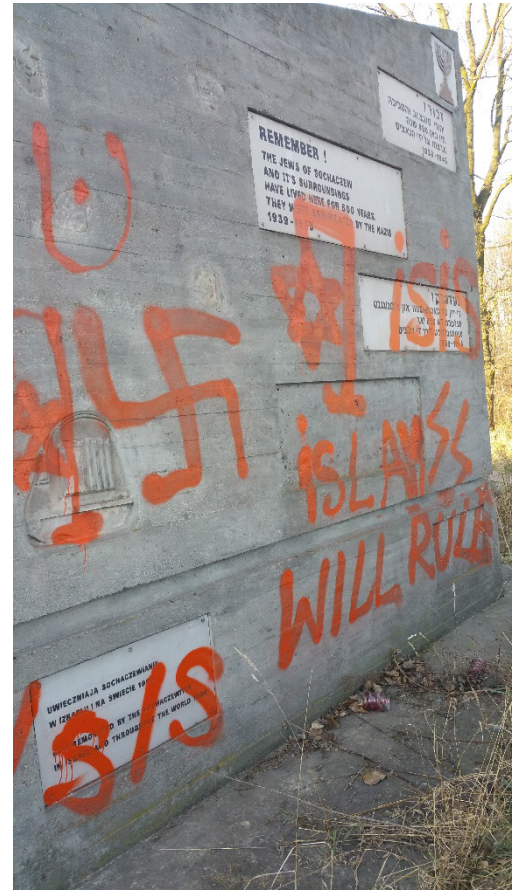
Figure 32. Graffiti on a Jewish cemetery monument in central Poland in 2018. The city officials and local police notified FODZ and quickly cleaned up the damage. The monument is behind a locked gate and substantial fence.
