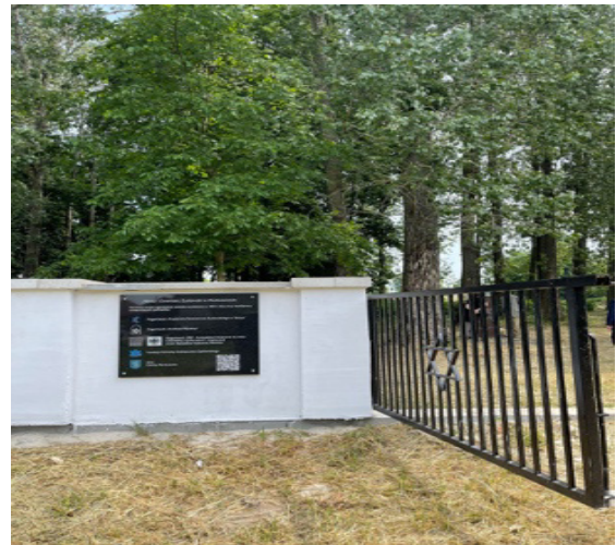
Figure 27. Markuszów Jewish Cemetery - new fence and wall around part of the cemetery; the remainder will be delimited with a plant hedge.
